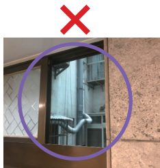
Failure to install screen windows
