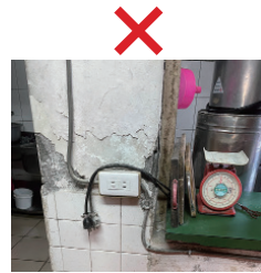
Peeling paint in places of operations
