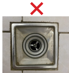
Lack of measures installed to prevent the invasion of vectors from drains
